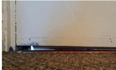
Fire door does not close properly or there is a large gap at the edges or underneath.
