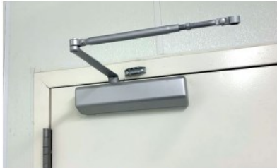
Door closer is broken or does not shut the fire door.
