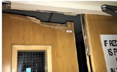
Fire door is damaged or has a hole in.
