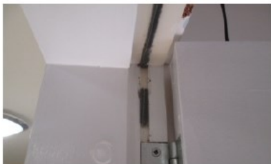
The seals around the edge of the door or frame are damaged, missing or have been painted over.
