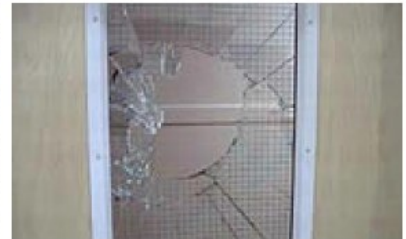
There is damage to the glass panel.
