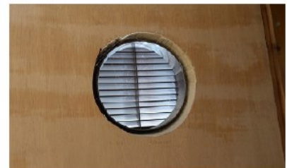
The fire door has had changes made to it after it was fitted, for example a ventilation grill has been added.
